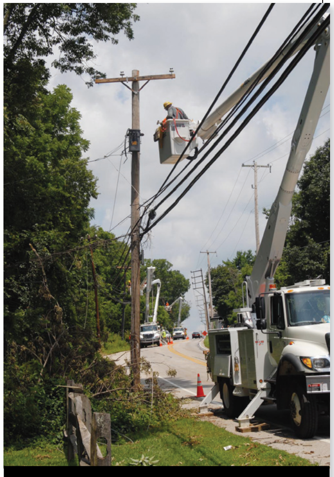
After a severe band of thunderstorms passed through southeast Pennsylvania and knocked out service to more than 400,000 customers, PECO operations personnel worked around the clock to repair the distribution network and restore electric service. PECO's AMR system helped ensure that the crews were dispatched to actual outage jobs.
