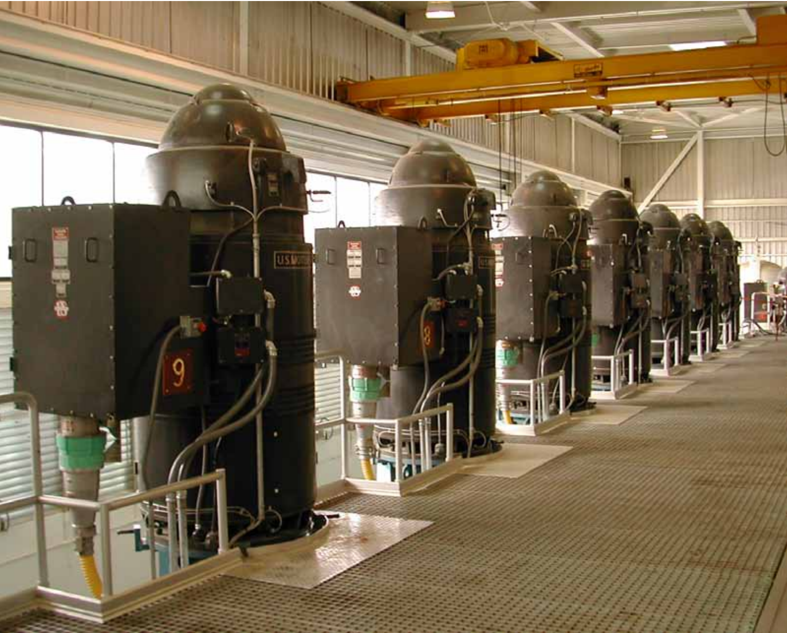
Large transmission pumps are major energy consumers. Black & Veatch
